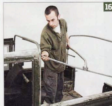
Now, the whole lot can be lifted into place and bolted to the hoops at either end.
